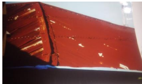
Fig. 4. Rusted roofing sheet
